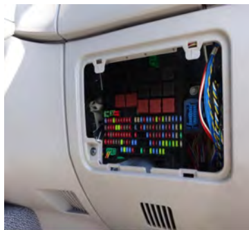
Figure 7-2.2 Inside View - Electrical Junction Box Location
